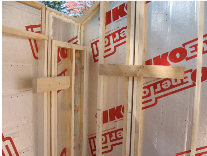
Figure 3-Assembled wall panel view from inside. Corner panel is one continuous unite to enhance the detail for the insulation and sealing.
